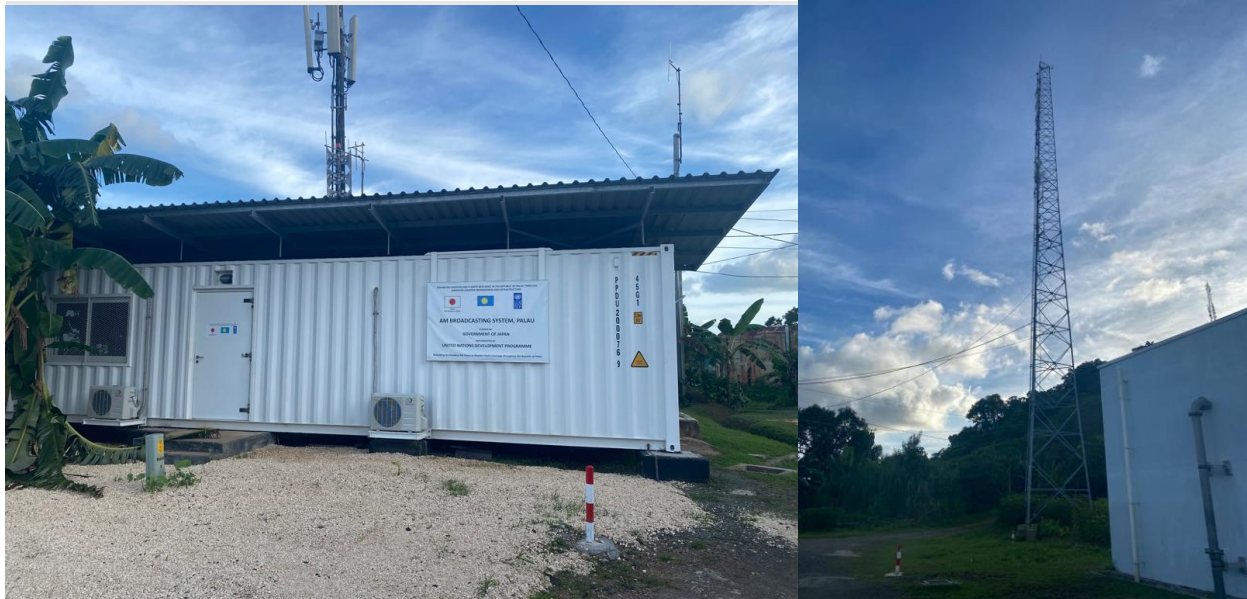
Figures 5 and 6: Equipment related to AM broadcasting system and antennae procured under Activity 1.5
